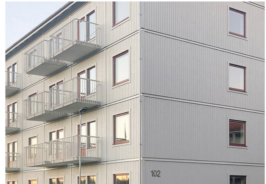
Fig 25) Visible horizontal seams between floors Project: Tega Ängar, Ytterby
