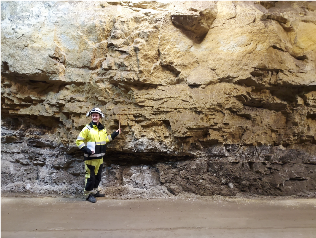
Figure C.3: Wall of a main corridor. Ruler is 60 cm for scale.
