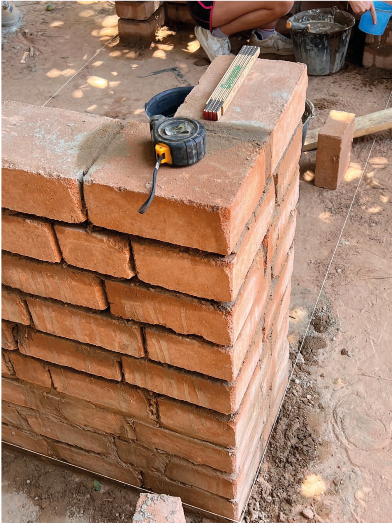
Wall is ready to cast the springer, concrete beam on which the vault will rest.
