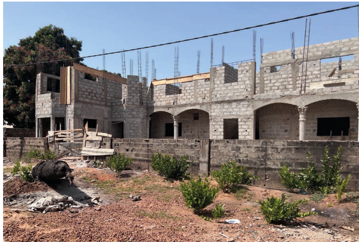
Structure built floor by floor, with concrete skeleton cast within the concrete blocks walls
