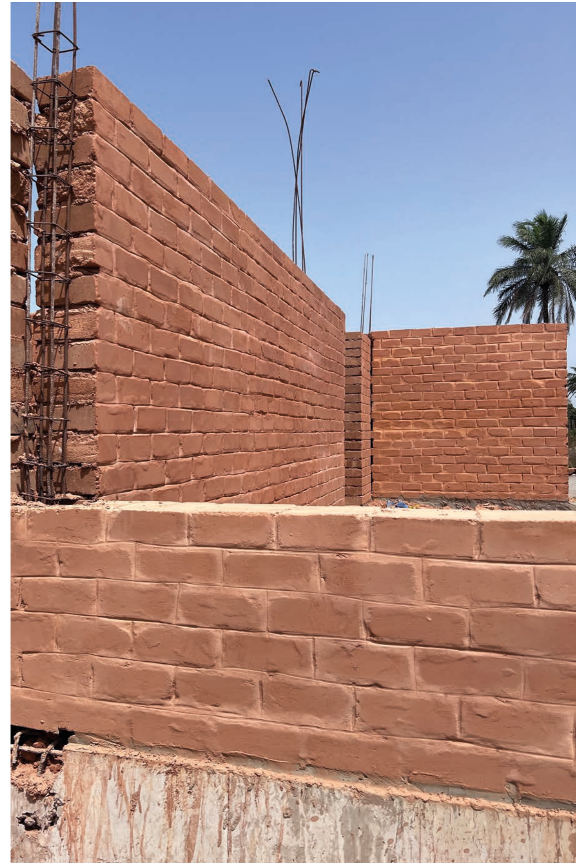
Construction site in Sanyang of Eco building construction showing the process of raising the walls to cast concrete structure within it.
