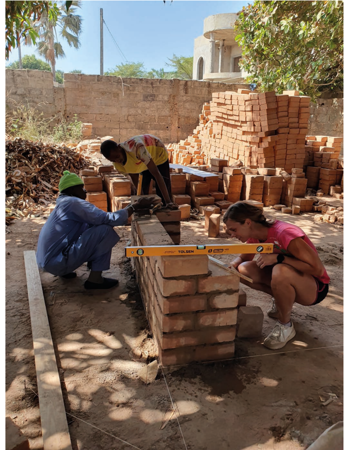
Building the walls on which the vault would stand. Blocks need to be leveled horizontally and vertically.
