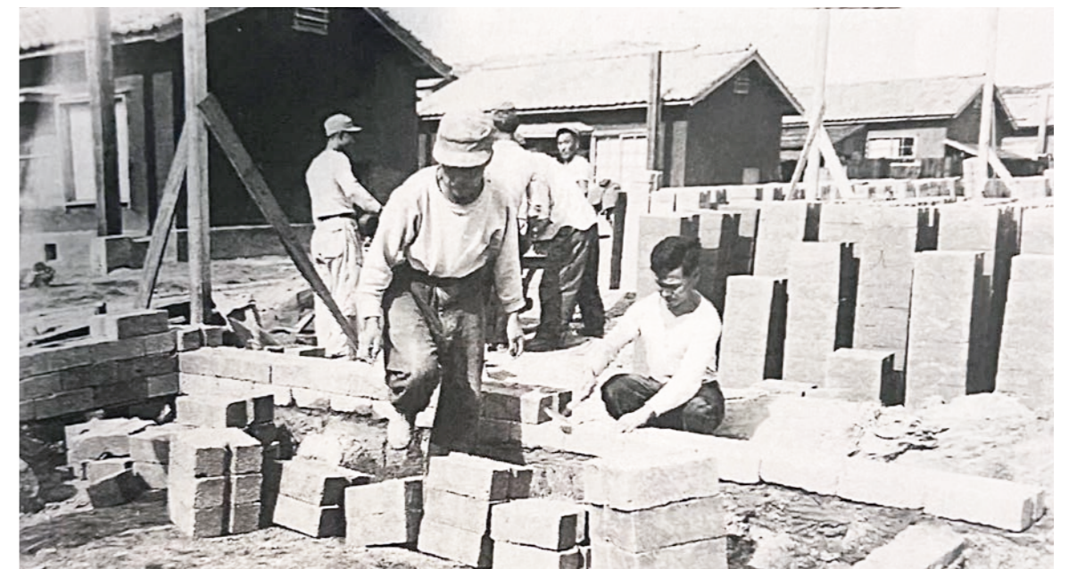
Workers laying rammed-earth blocks at UNKRA (United Nations Korea Reconstruction Agency) housing in South Korea following the Korean war 1950-1953 (UN Photo Archives)
