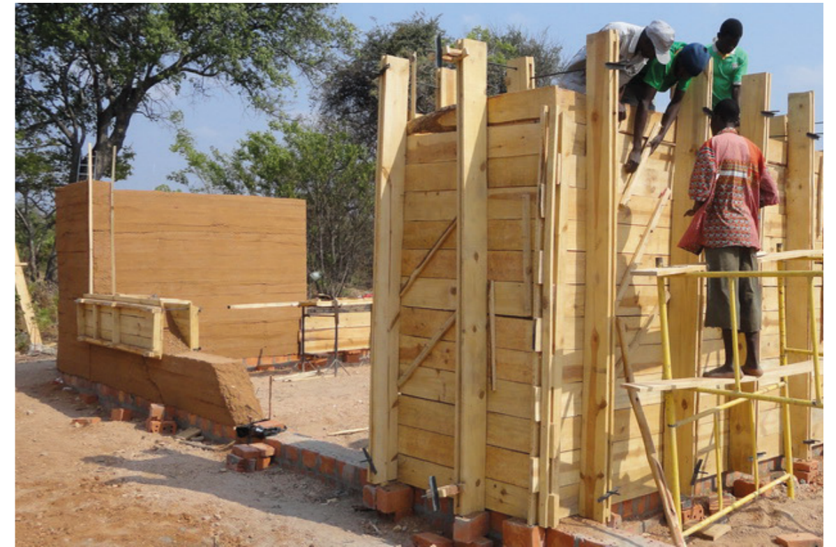
Moving and fixed formwork in rammed earth project, Zambia (Rammed earth consulting, n.d.)
