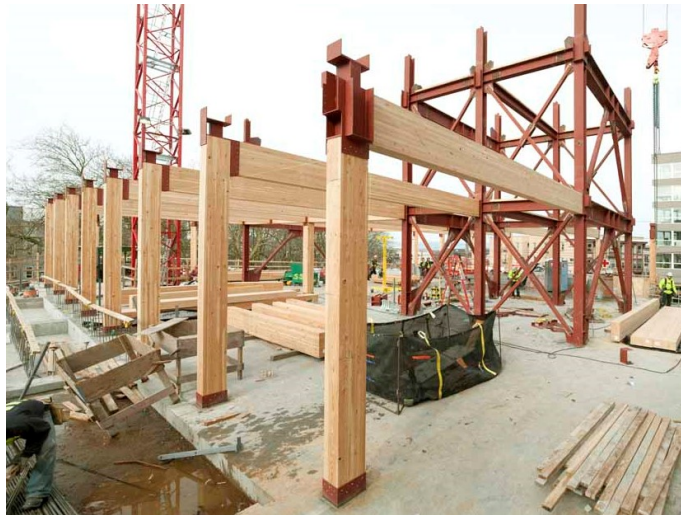
Figure 2.6: Construction of a timber frame system used in Bullit Center, Seattle, USA. The glulam columns and beams are connected to a diagonally braced steel frame core (Stamets 2012).
