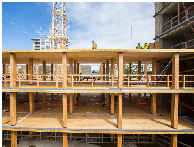
Figure 2.8: Hybrid system of Brock Commons Tallwood house, Vancouver, Canada. CLT floors and glulam columns are braced by concrete cores (Credit: naturallywood.com, photographer: KK Law).
