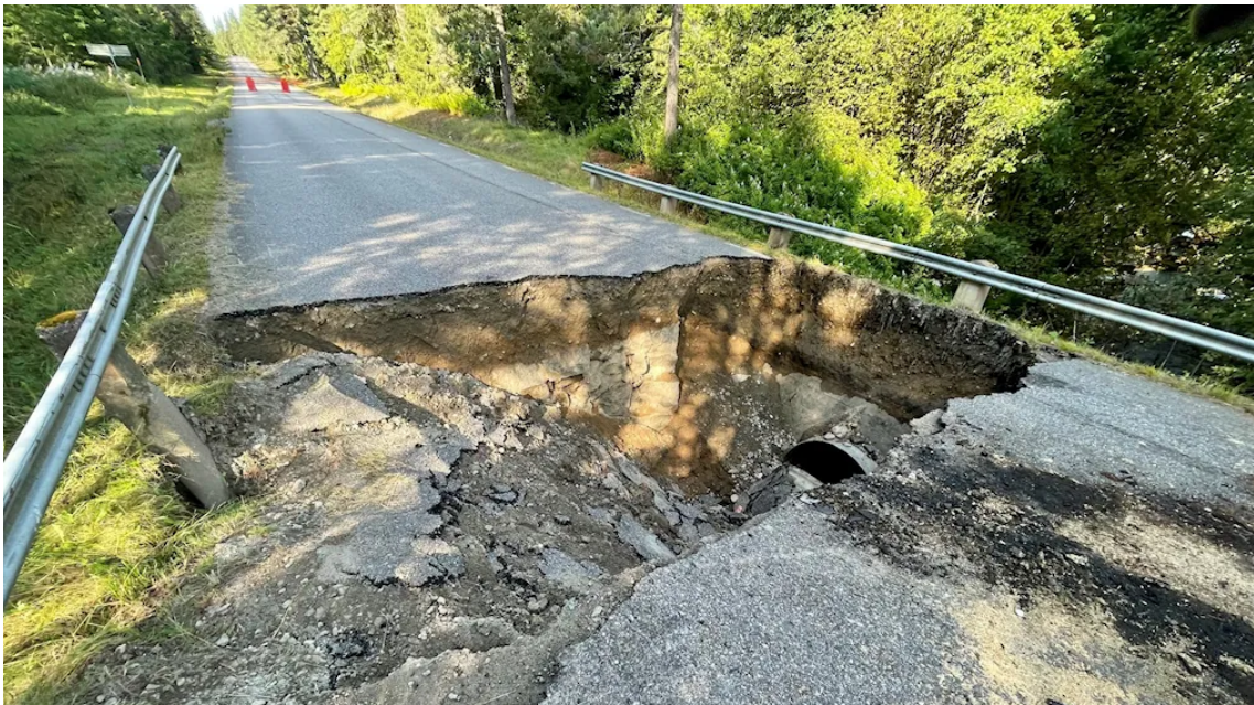
Figure 3.3: Picture of the flushed away road embankment in Brattfors. Reprinted with permission from P4 Gävleborg/Sveriges Radio (2021).
