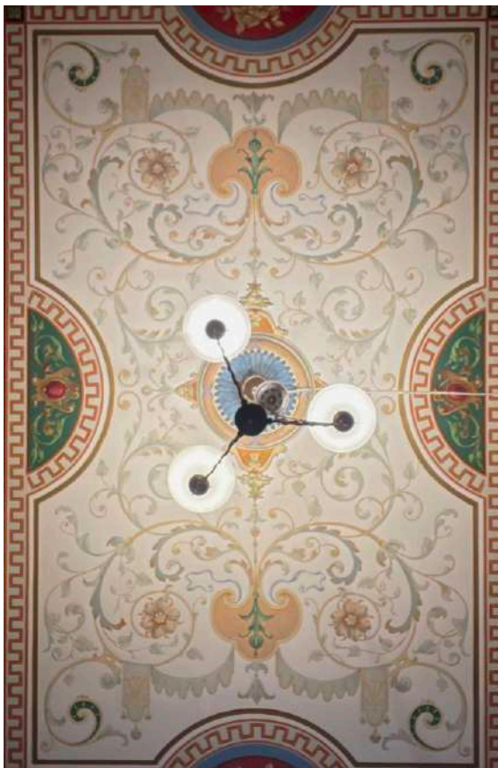
Image 30. Wall painting at the ceiling.
