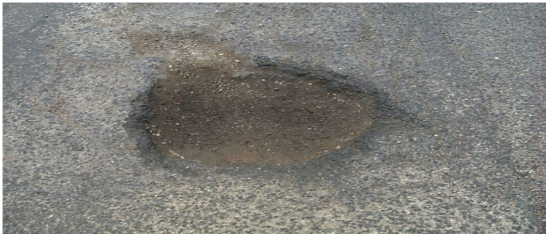
Figure 3.5 Pothole formed on the bridge deck slab
