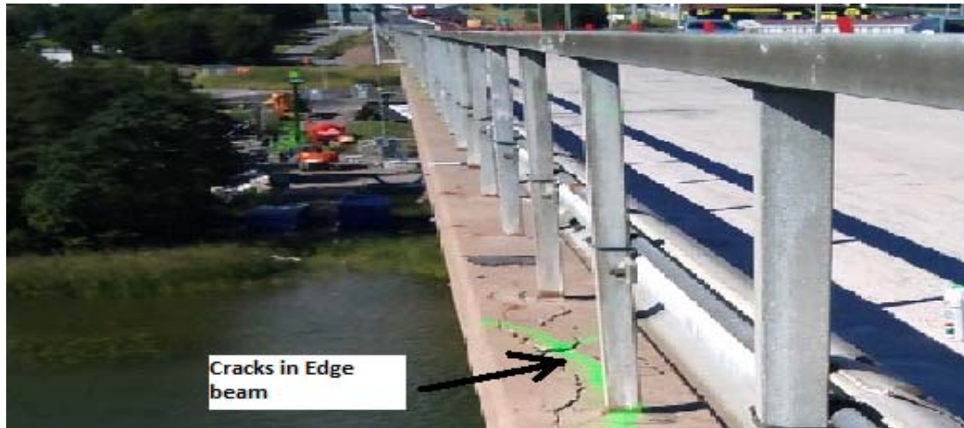
Figure 3.6 Cracks in Edge beam
