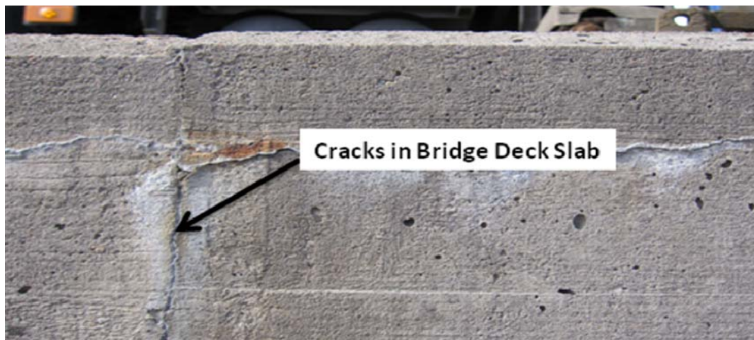
Figure 3.1. Cracks in bridge deck slab
