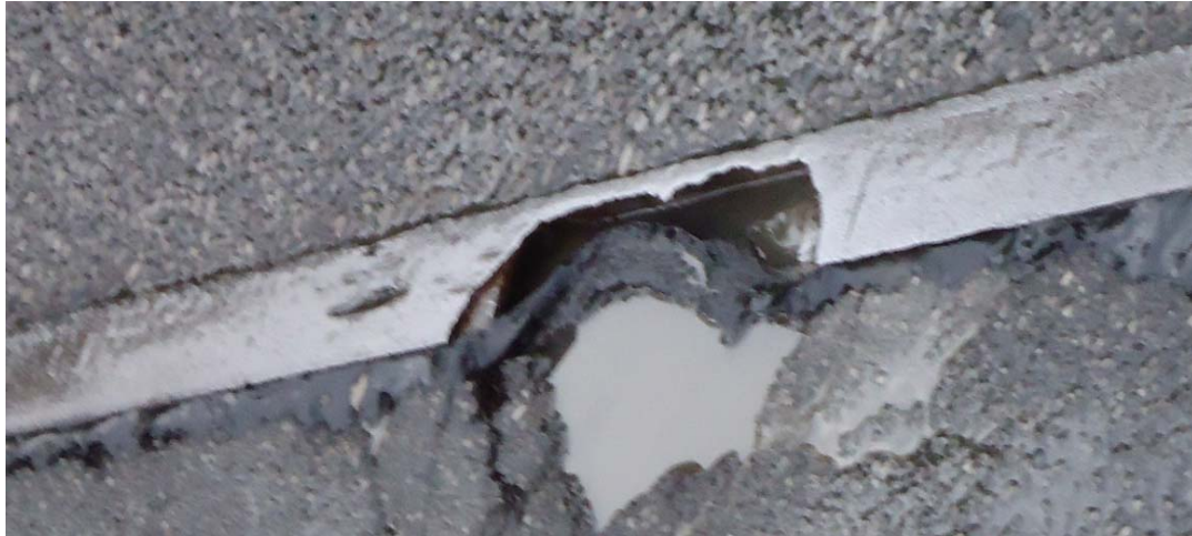
Figure 3.7 Damaged expansion joint
