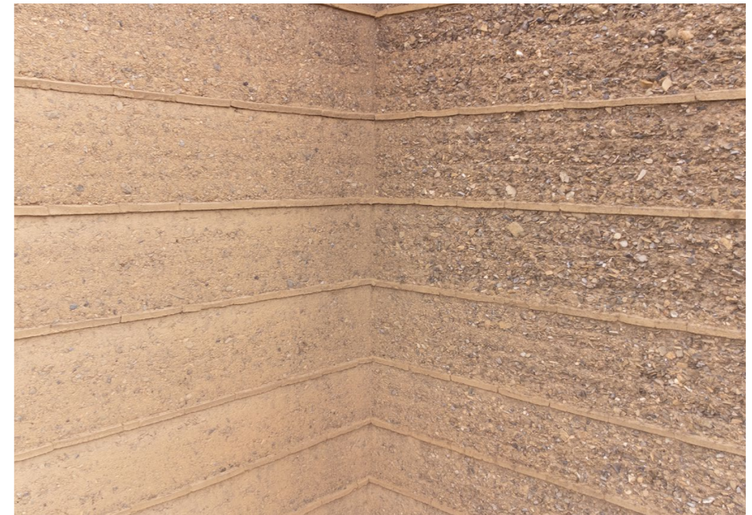
Figure 65. The general wind direction has caused more erosion on one side of the facade. Haus Rauch, Schlins.
