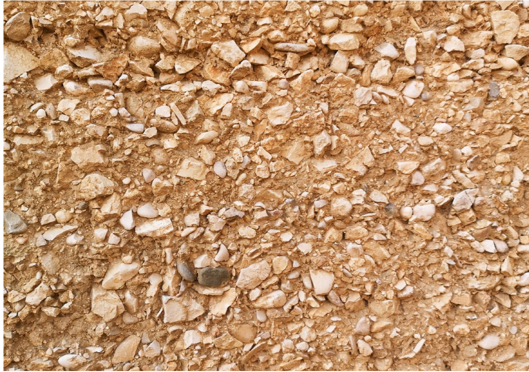
Figure 62. Exposed brighter stones on the eroded facade. Swiss Ornithological Centre, Sempach.
