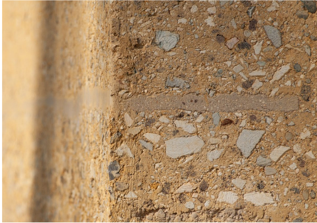
Figure 72. Where the elements have been cut the stones and erosion checks are also cut straight. Alnatura Campus, Darmstadt.
