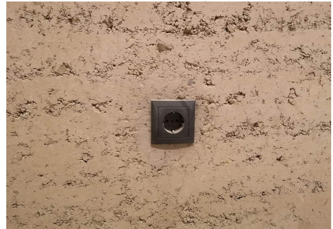
Figure 86. Yes, it is possible to have power sockets and other installations in a rammed earth wall. Erden Werkhalle, Schlins.
