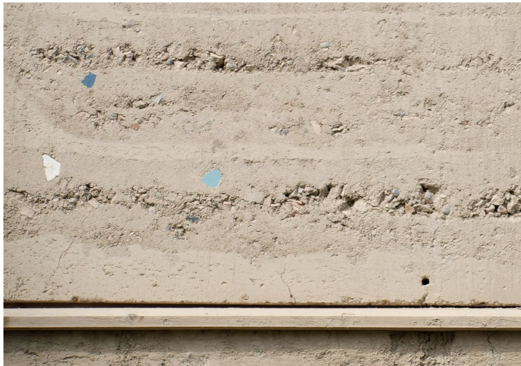
Figure 88. Remnants from a demolished house have been mixed with the earth. Kiln Tower, Cham.
