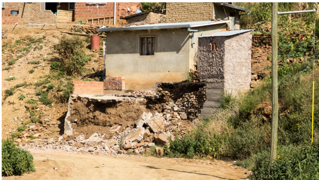
Figure 6.1 A construction which has been damaged due to the unstable ground (Photo: private)
