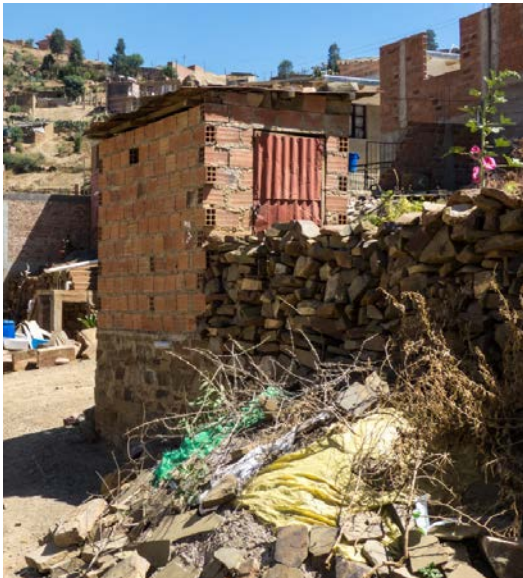
Figure 6.6 This is how a pour-flush toilet right above an improved pit can look from outside (Photo: private)
