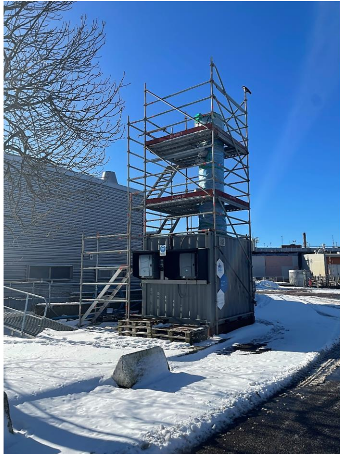
Figure 3. AGS pilot plant at the Rya WWTP.
