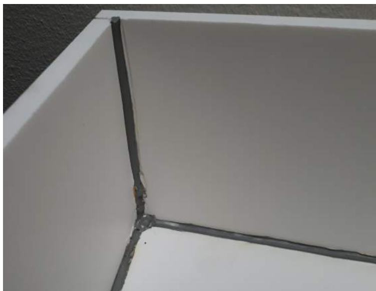
(b) The weld joint.
