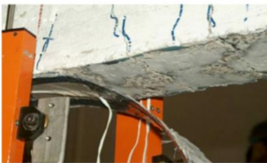
Fig : 12 Debonding of FRP laminate [20]
