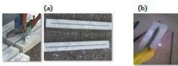
Fig -4: (a) Cutting of grooves and (b) filling of grooves with epoxy
