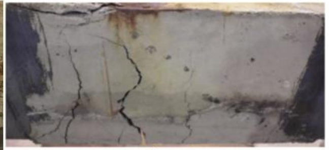
Fig: 11 Rupture of corrosed tensile bar back face crack[42]
