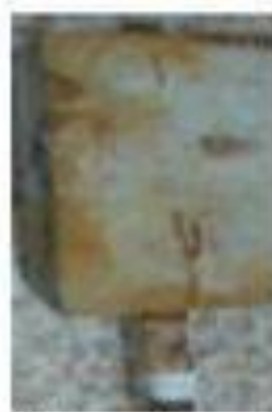
(a) pullout failure
