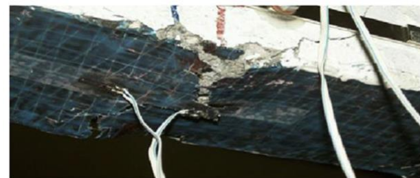
Fig : 13 FRP laminate rupture[20]
