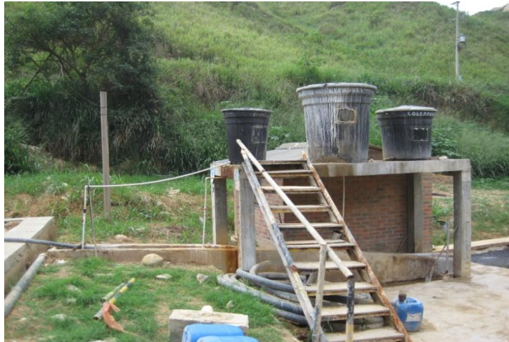
Figure 8. Chemical treatment of the leachates in the landfill.
