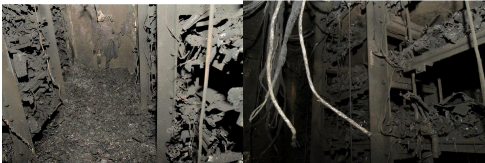
Figure 10 Damage to the battery room, seen from the left to right: battery stacks.[27]
