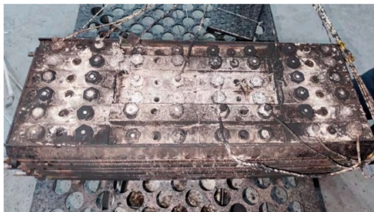
Figure 29 Picture of the LIB pack after the combustion test.[36]
