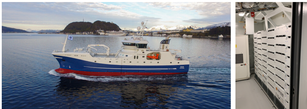
Figure 3 Below-Deck Corvus Battery Bank on Longliner Geir with Forced-Air Cooling. [10]
