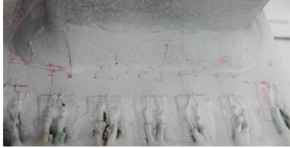
Figure 3: The difficulty to distinguish fatigue cracks from scratches after dye penetrant is applied
