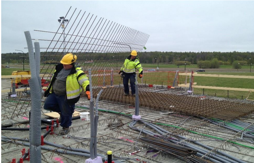
Figure 4.10 removing and relocating reinforcement during material delays delivery Source: Botrygg, Örebro ,Fallskärmen residential project
