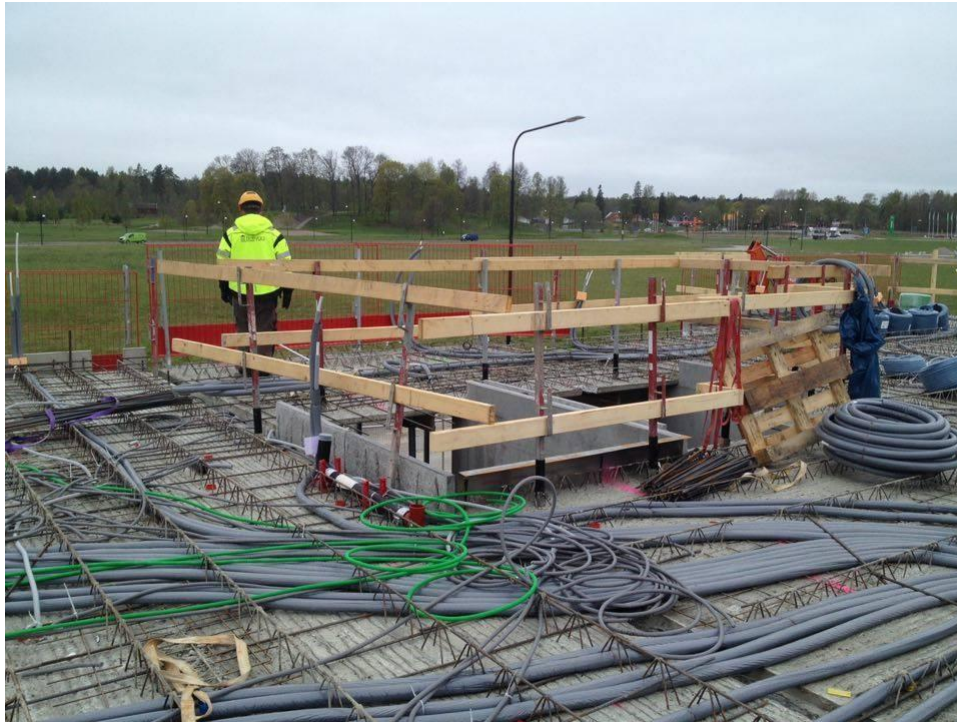
Figure 4.9 Gaps in the slab which became reinforced at a later stage in a rework. Source: Botrygg Fallskärmen residential project in Örebro.
