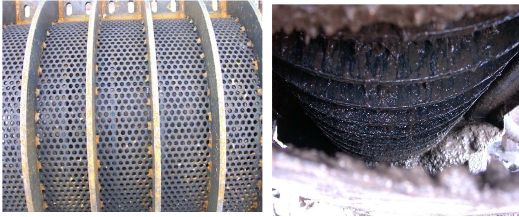
Figure 4.3 Filter separating feedstock to compost and to biogas plant. Right picture is taken when filter is under operation.
