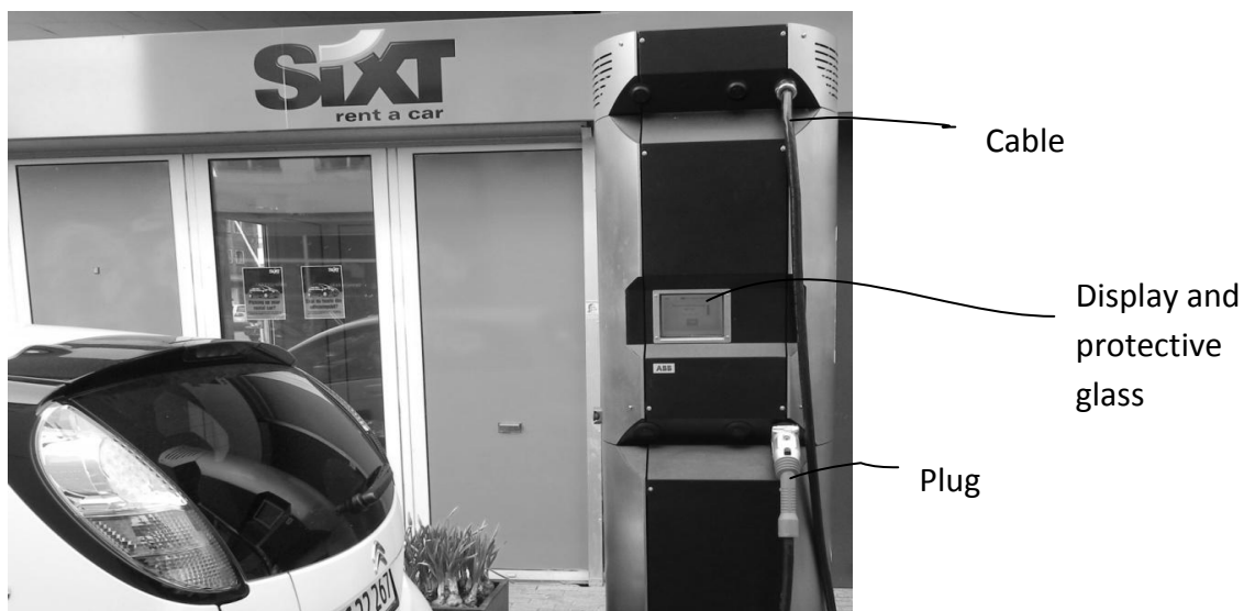
Figure 35. The DC Fast Charging prototype installation in Copenhagen. The picture also shows the components that are subject to wear and tear (author).
