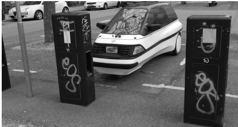
Figure 34. AC Slow Chargers installed 20 meters from the DC fast charger in Copenhagen (no security cameras for protection) (author).
