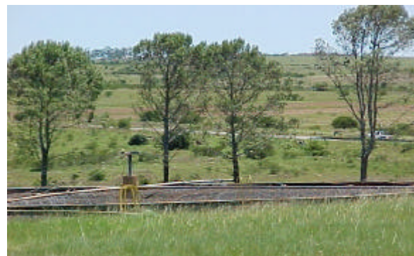
Figure 19 Biological filter unit at Shornville Sewage Treatment Works.
