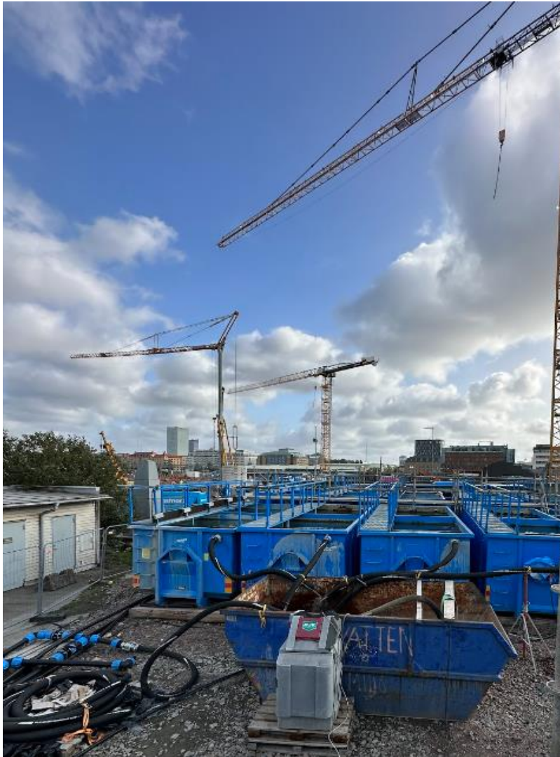
Figure 7. Illustration of the treatment system for the excess tunnelling water on site (Photo by F. Hadi).
