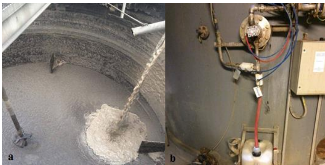
Figure 12 a) 809 vessel from a view above and b) the drain crane for the R4 vessel.
