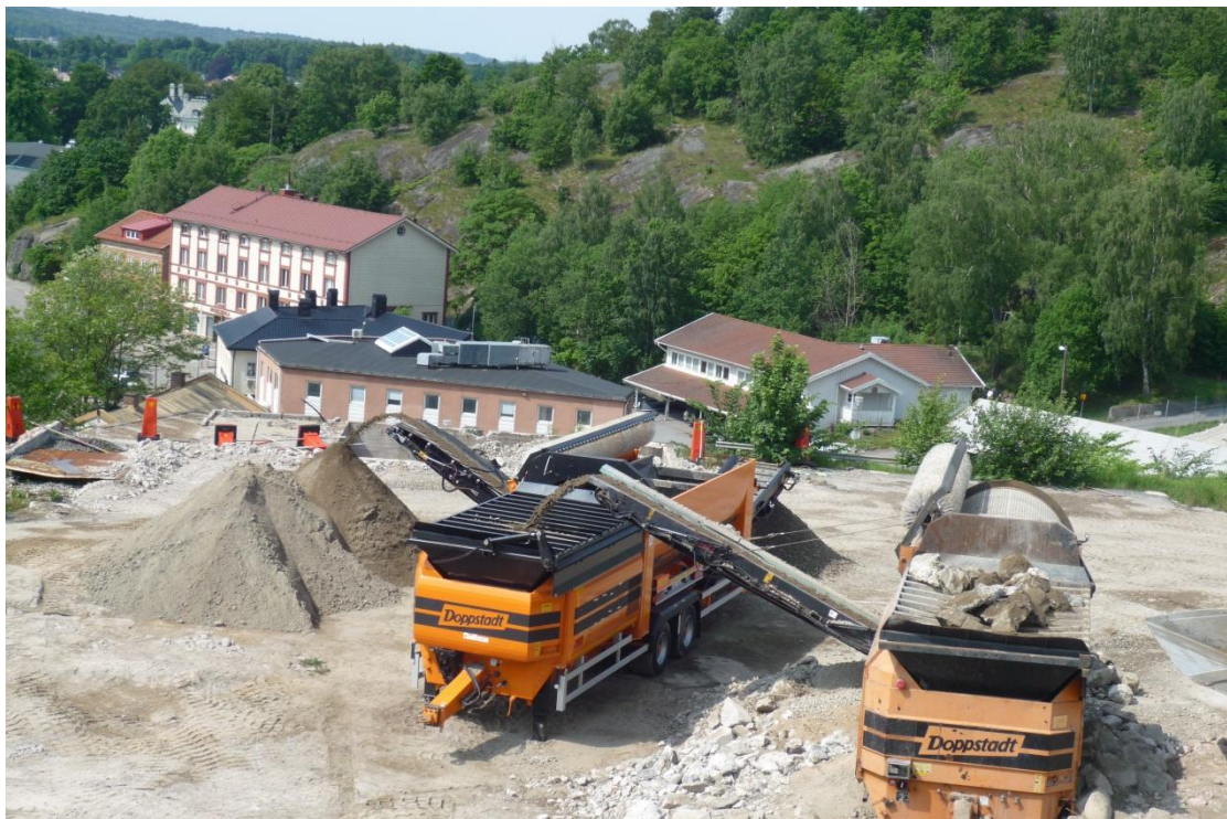
Figure 5.4. Overview of the sieving process at Hexion. Trammel screen to the right and star screen to the left. Photo: Åsa Landström.
