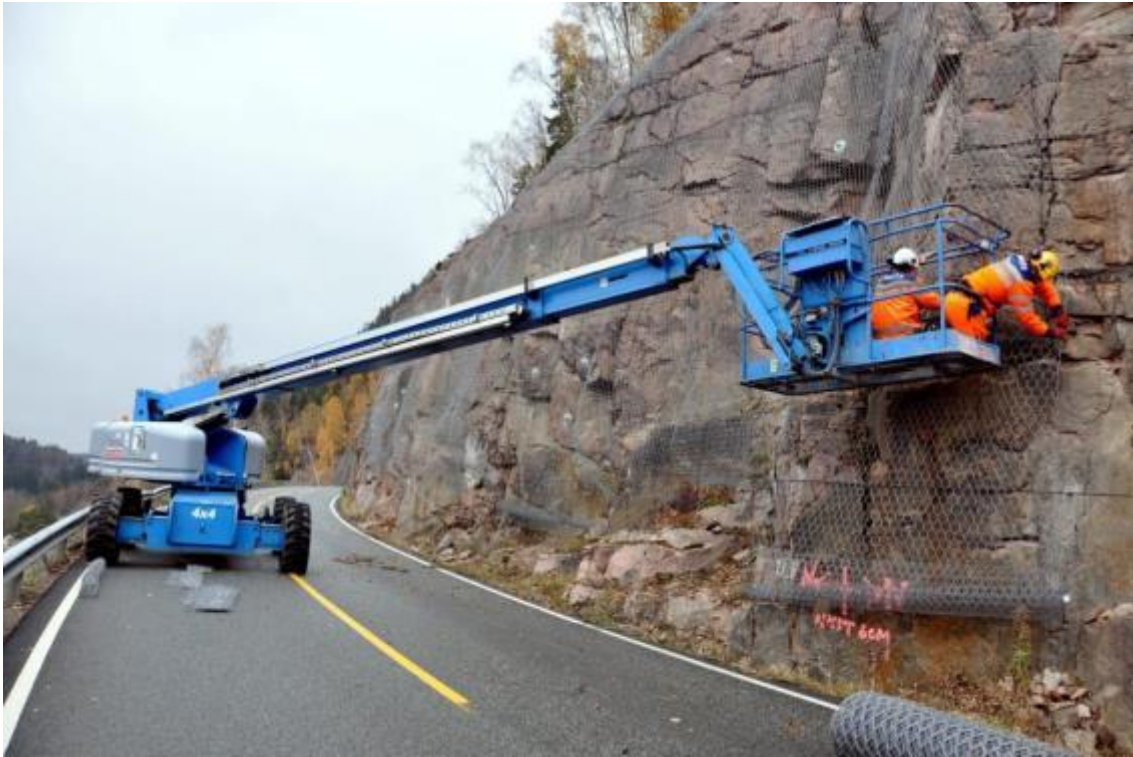
Figure 29: Mounting of rock safety net along Grimsrud road in Hurums municipality, Norway. The net is identical to the one used for securing ice (Royken og Hurums Avis. 2010).
