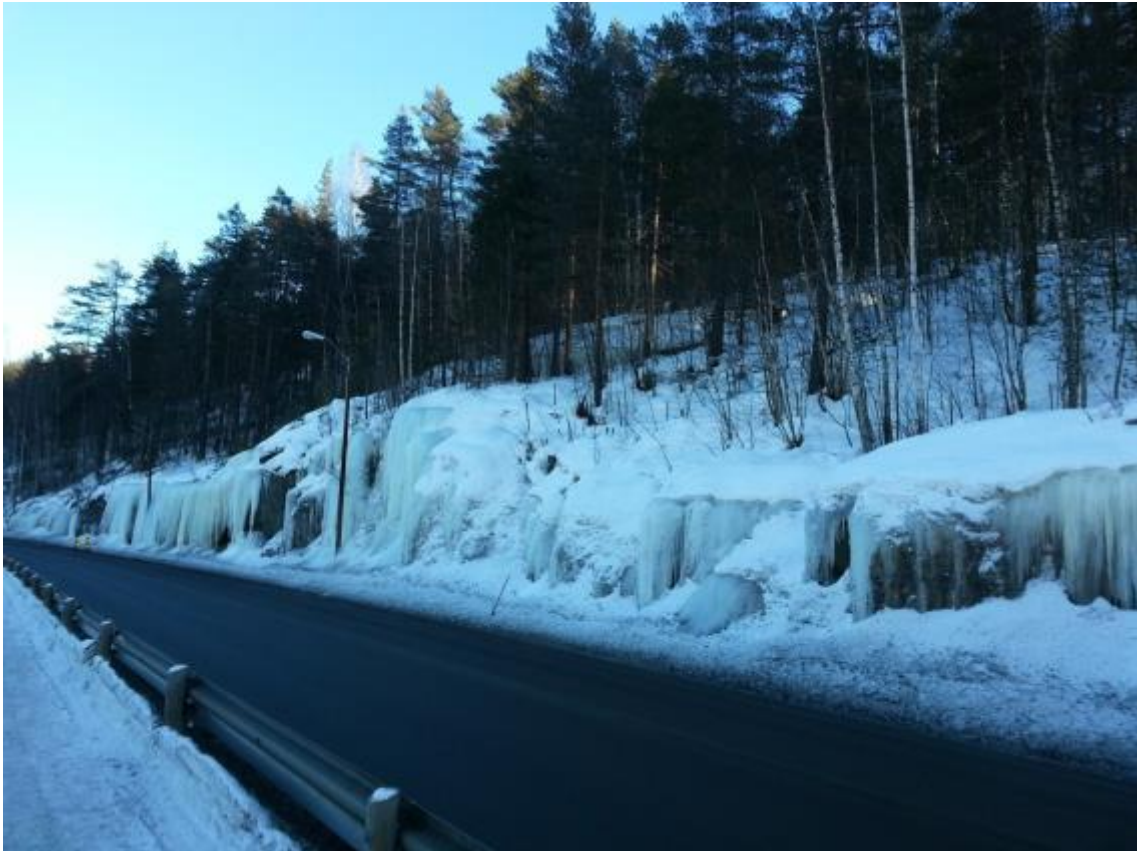
Figure 10: The existing rock cut during a site visit on the 25 th of January 2013. This picture was taken 13:29 so it's clear that the sun does not shine in the study area some part of the winter.
