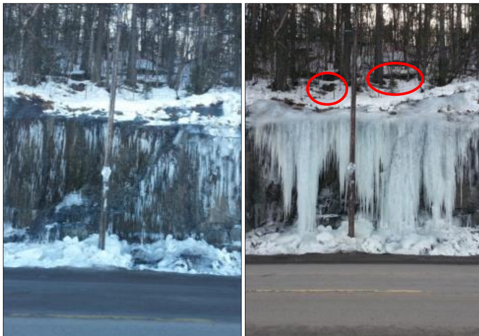
Figure 12: On the left is the existing rock cut the day after the ice was removed. The picture on the right is the same location 5 days later. The rock was notably wet under the removed ice.
