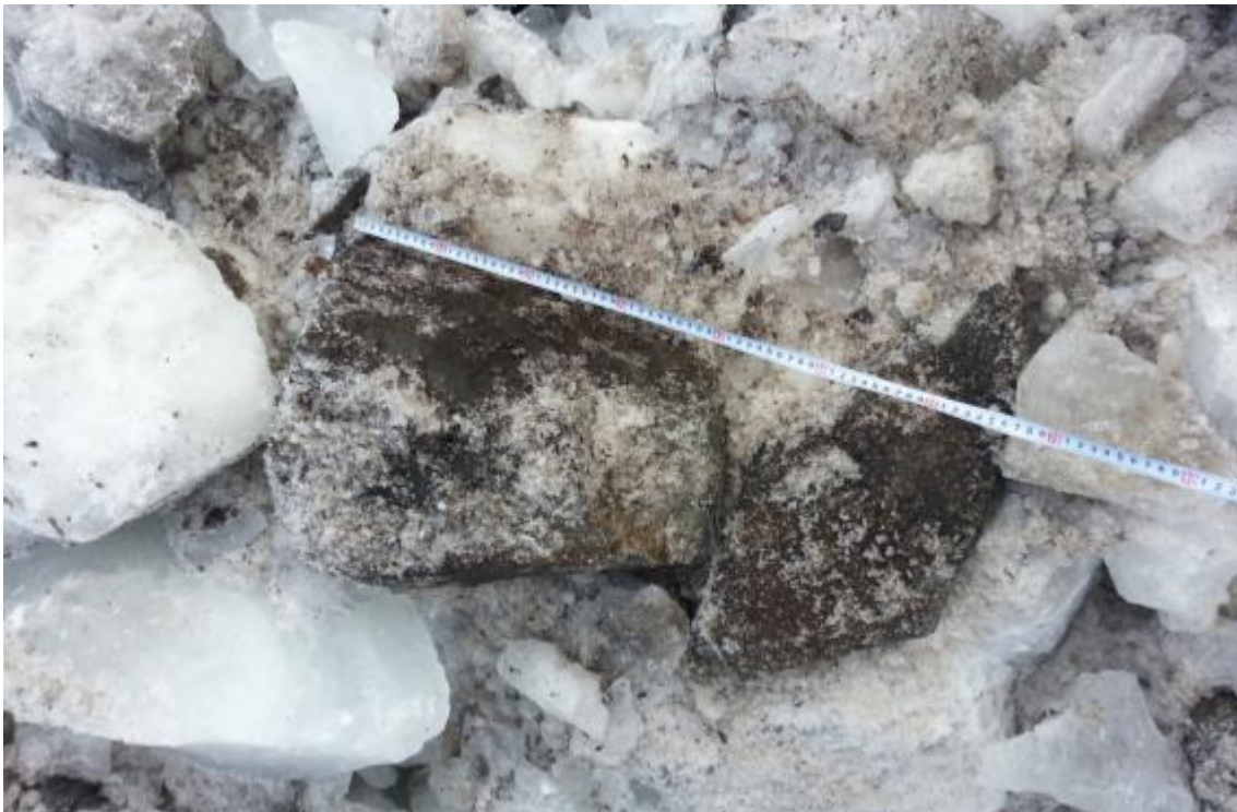
Figure 24: This stone block was stuck in the ice removed from the rock cut in the study area. It is around 65cm across.
