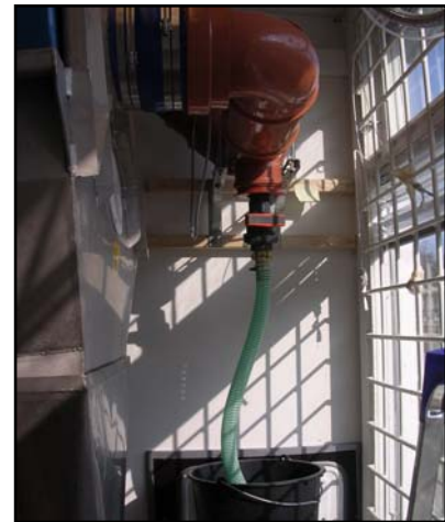
Figure 11. Inlet for black water sewage into the drum screen
