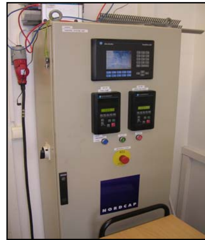
Figure 14. A PLC (Program Logic Controller) is controlling the whole process.
