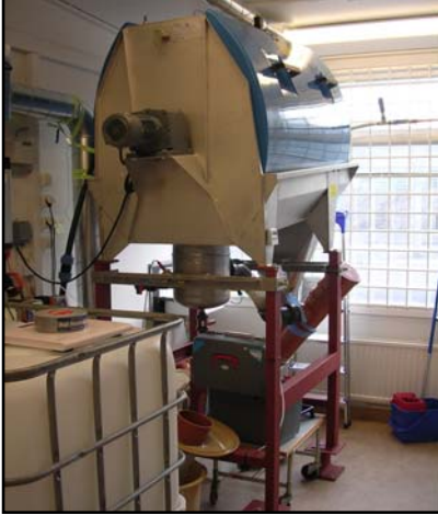
Figure 10. Rotary drum screen operated to separate solids from the black water.
