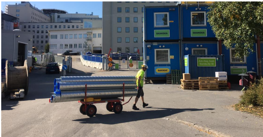
Figure 41: Ventilation parts that has arrived at NUS
