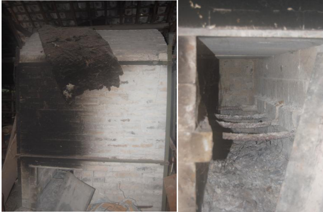
Figure 2: The furnace from the side. To the left, the furnace with the fire placement, and to the right, close up from the fireplace.
