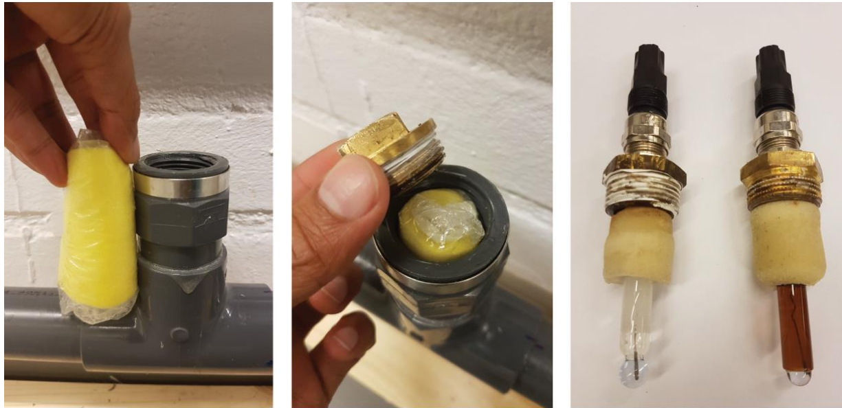
Figure 12: Using sponge for avoiding the stagnation of water and air in the nodal junctions.
