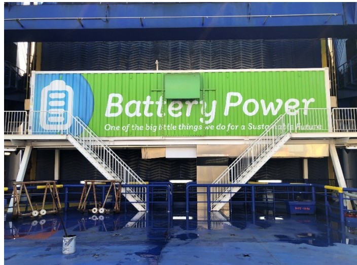
Figure 9. Shipping container housing the batteries (Authors own copyright)
