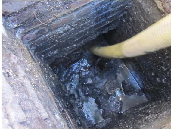
The hose is connected to the beginning of the septic tank.
