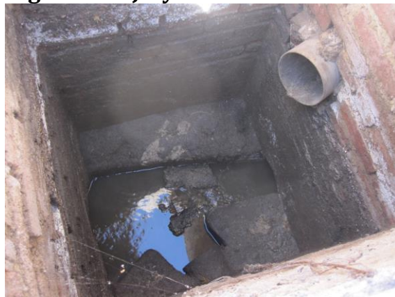
Very low water level at point 2.
