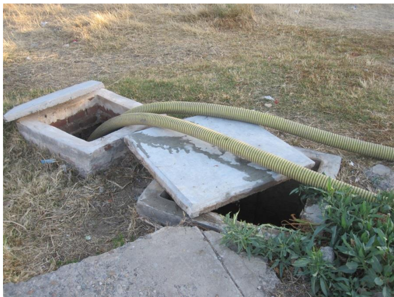
Picture 4. Maintenance with ServiMaster. The entrance to the septic tank is located to the left in the picture and point 1 is located to the right.
